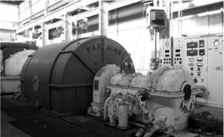
Parsons turbo-generator set in the power station, Pyestock Image © Simon Cornwell
