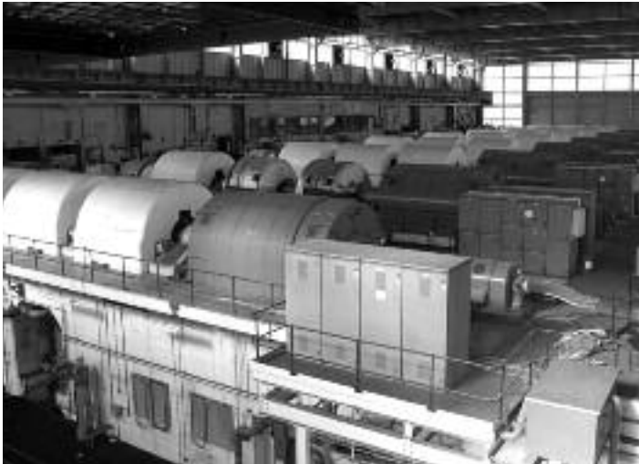
Main photo: Three drum boiler in Battle Test House
